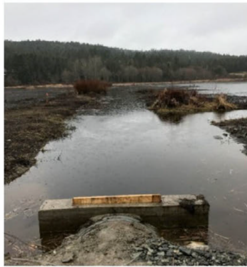
Channel, berm and headwall
